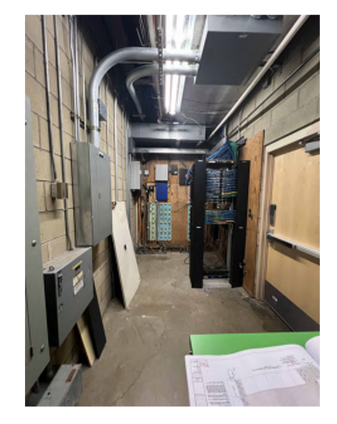
3 ELEC ROOM 1428 EXISTING RACK PHOTOS NTS
